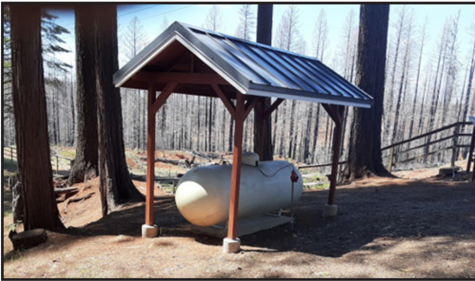
Liquid Propane Gas (LPG) storage tank
